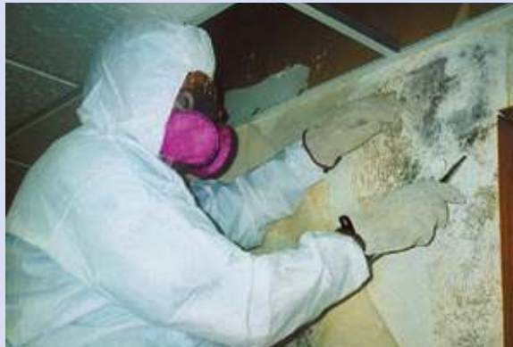
Photo 7: Remediation worker with limited PPE
