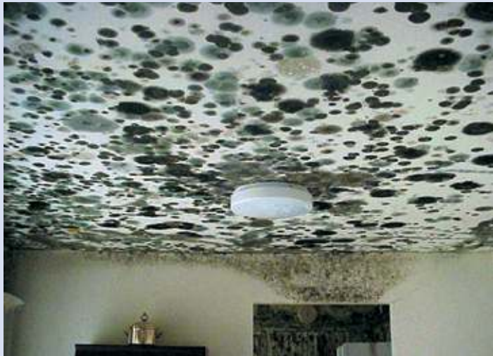
Photo 2: Extensive mold contamination of ceiling and walls
