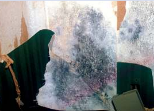
Photo 5: Mold growth behind wallpaper
