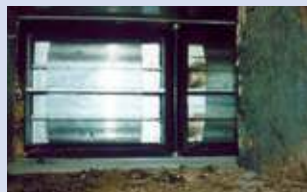
Photo 4C: Moldy air duct
